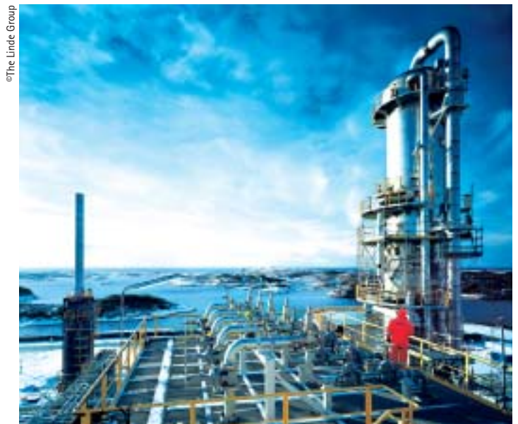
Innovative plant technology for the production of liquefied petroleum gas (LPG) in the Kollsnes gas processing plant in Norway
