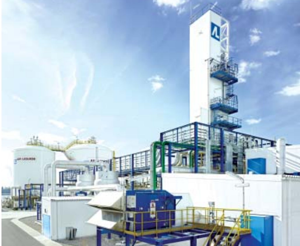
Air Liquide – the world leader in gases for industry, health and environmental protection – started the operation of a new air separation plant in January in Gundelfingen in the State of Baden-Württemberg. With the system round up to 700 tons of liquefied gases are daily produced from the ambient air.
